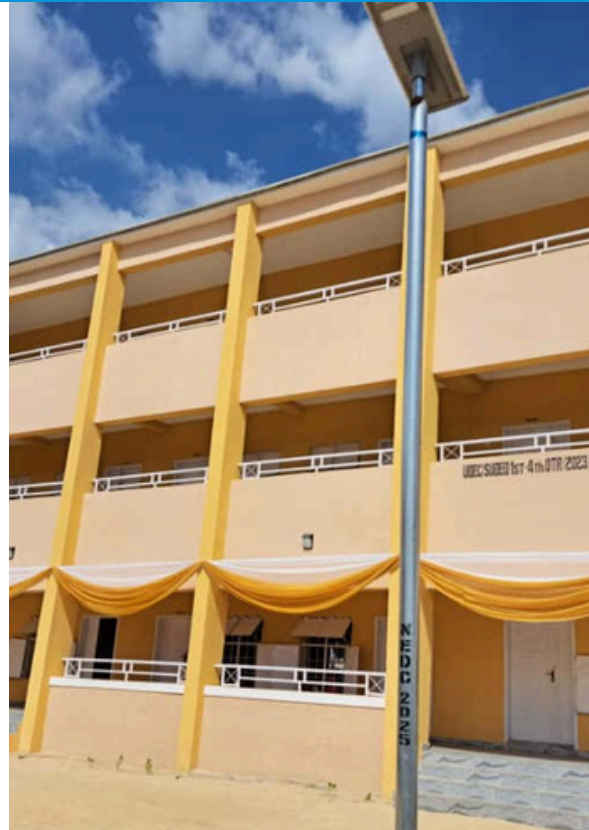
Newly renovated blocks of classroom by AGILE Project at Government Secondary School, Taban Sani, Kaduna.
