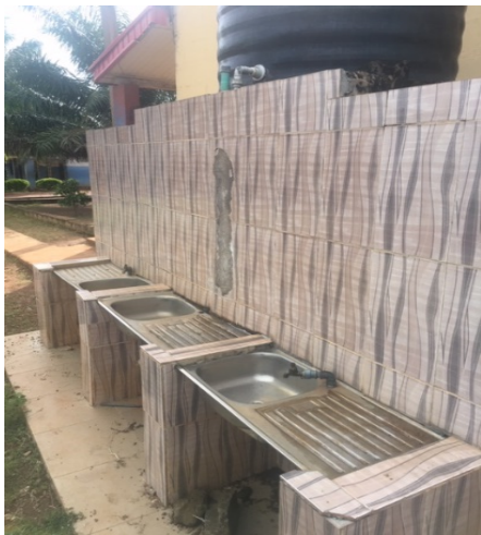
Plates 10: Hand washing facility for girls within the classroom area
