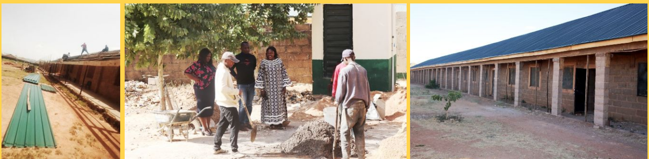
Ongoing construction and renovation of classroom blocks and toilets in schools around Plateau State.
