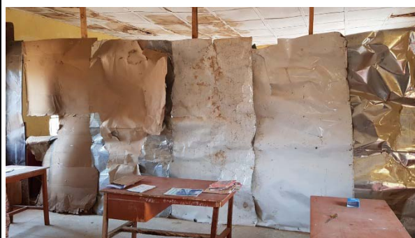
Plates 11: Use of zinc as classroom partition which emits heat thereby making the classroom inconducive and exposes the girls to injuries and tetanus from sharp edges
