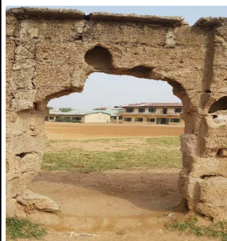
Plates 8: Broken fence which poses security challenge to the school
